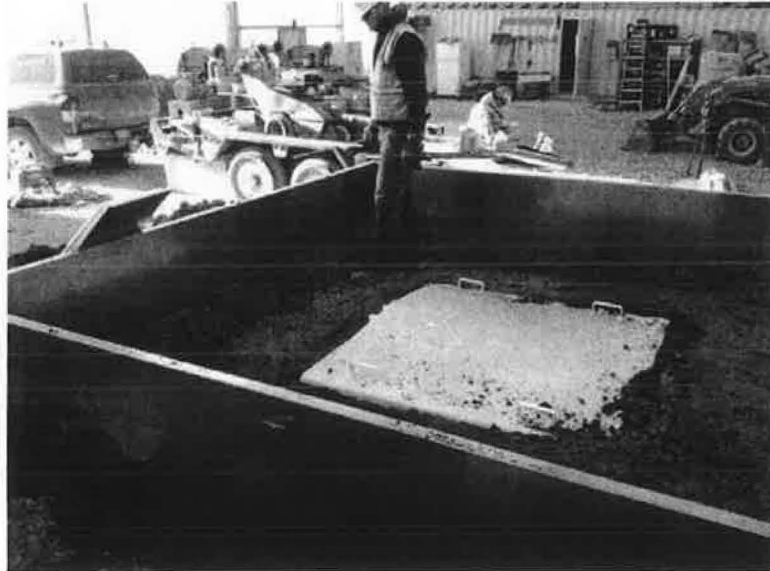
Figure 16 - SDRI with berms built on the inside around the periphery of the outer ring
