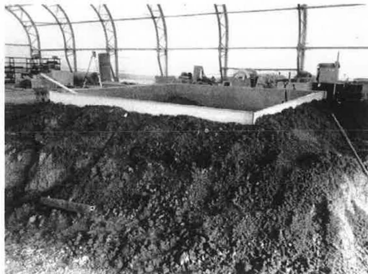
Figure 17 – SDRI with berms built on the outside around the periphery of the outer ring
